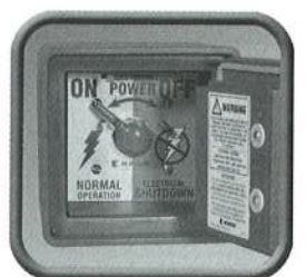
Power Shutdown Station
